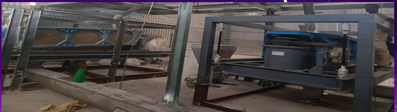
Two SHIVRAX sieving machines installed in Gujarat, India
